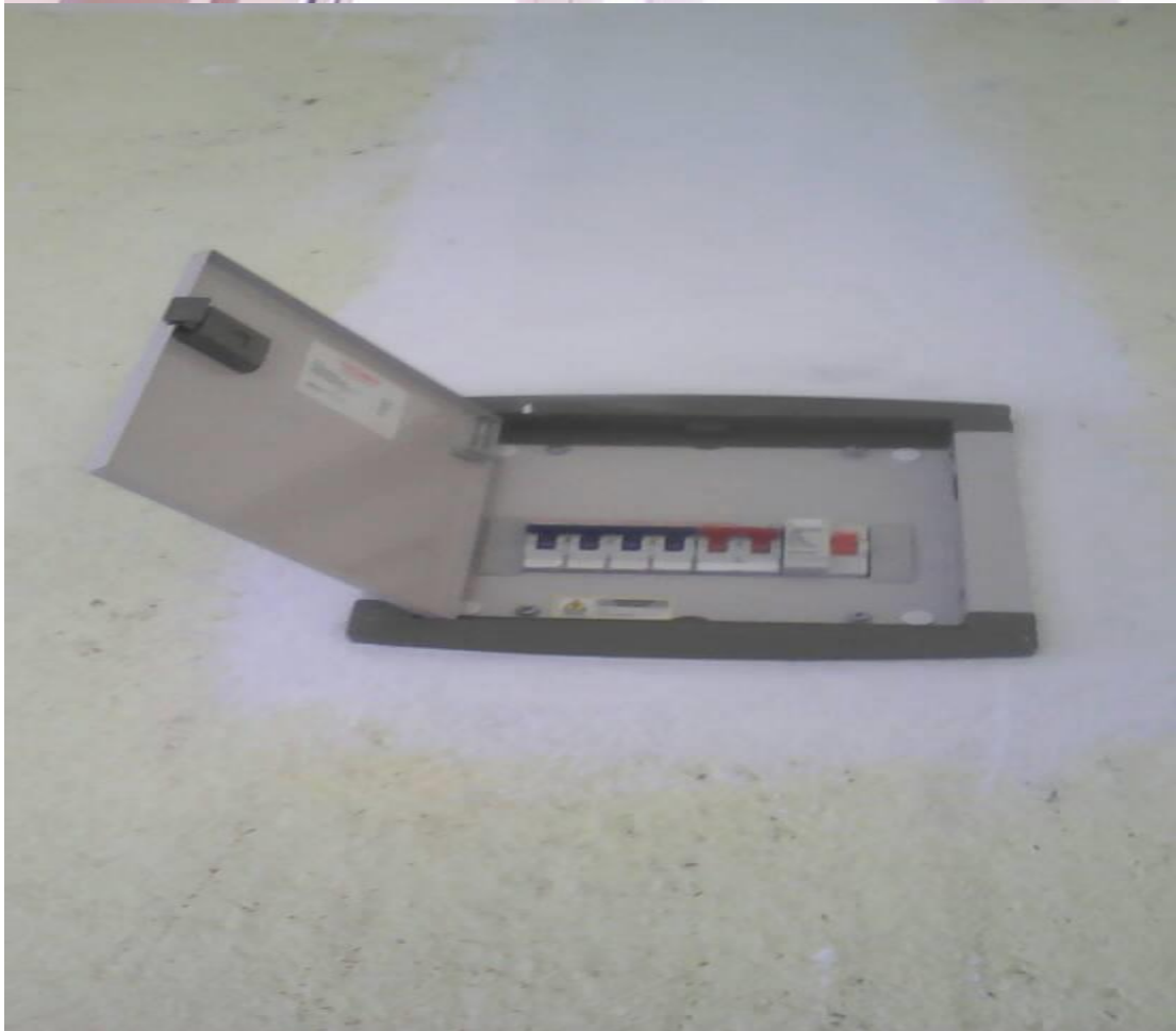
Electric Meter & Hallway corridor (wiring system is tested, safe and read to connect!)
